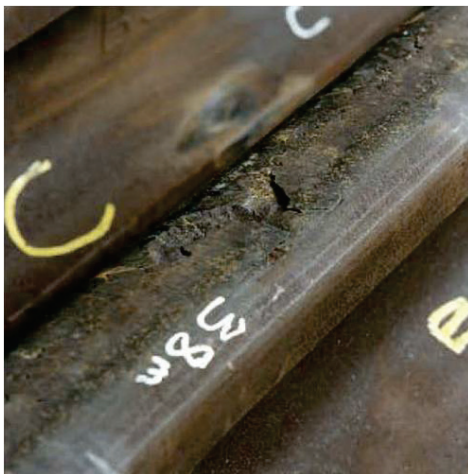
Fig. 1.34 Rail crown surface at the accident point (Spalling) [22]
