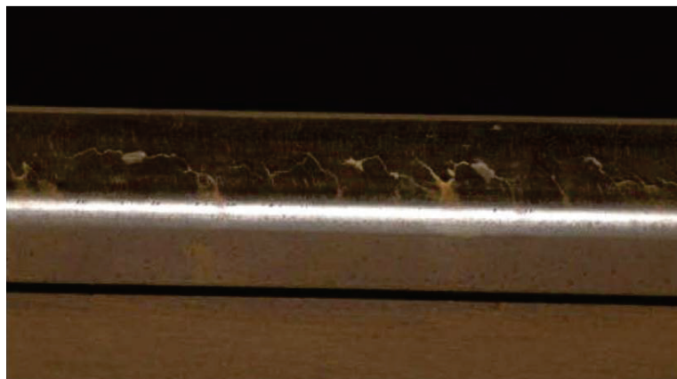
Fig. 1.33 Rail crown surface at the accident point (Gage corner cracking) [22]
