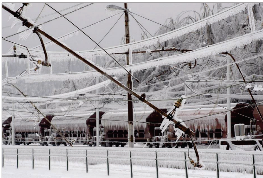
Fig. 1-9 Electric Wire Icing (12)
